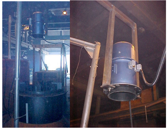
Figure 20. Views of sensor, electrode casing and casing measurement pointer mounted on electrode galls.
