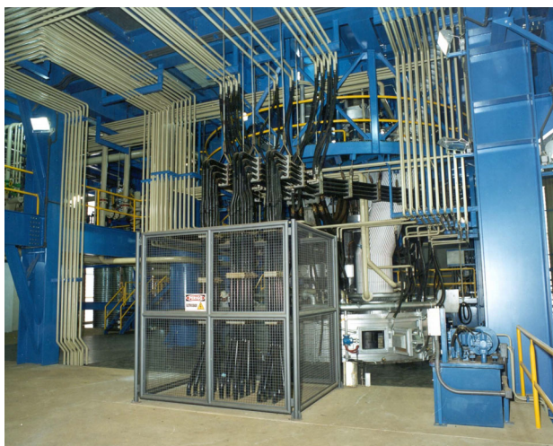
Figure 9. Dephosphorization furnace for the ferro niobium industry.
