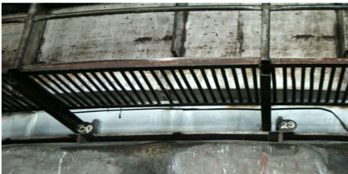
Figure 1: Furnace bottom cooling air outlet
