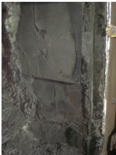
Figure 6: Crack on big block lining on ferromanganese furnace
