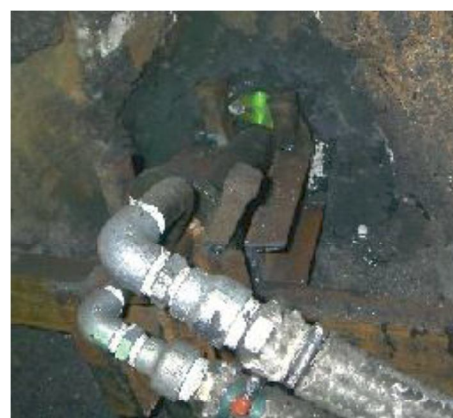
Figure 8: Water-cooled copper tube in the tap hole
