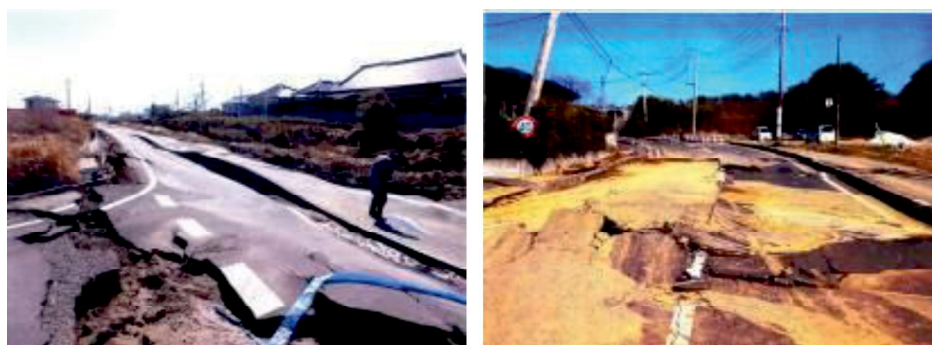
Figure 3.1.1: Uplift and caving-in caused by liquefaction
