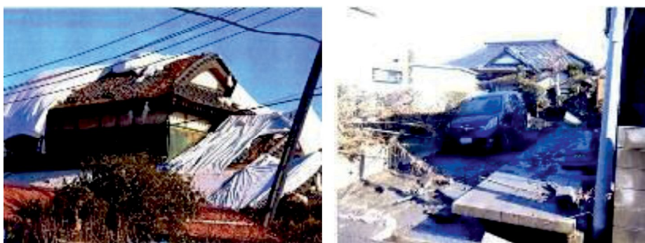
Figure 3.1.2: Damage to roofs and walls
