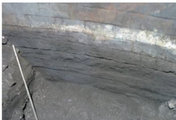
Figure 4: Condition of Sidewalls after four years of Operation
