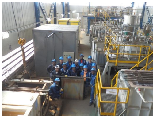
Figure 11: EMM Pilot plant – First production – July 2013
