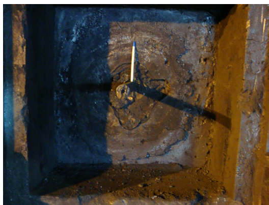
Figure 14: Tap-hole condition observed during TPS-2012 (after 11 years of service)
