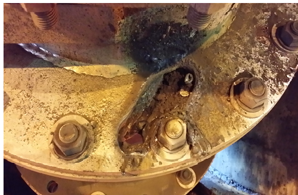
Figure 16: Arcing of feed chute due to material leakage
